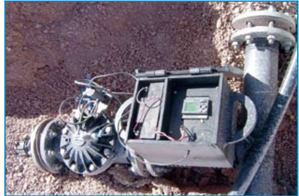
Electric valve, controlled locally
