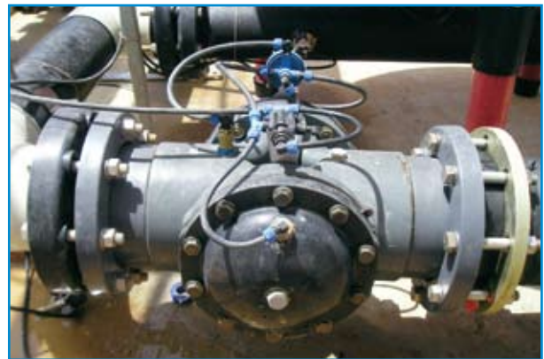
Pressure Reducing valve, remotely-controlled
